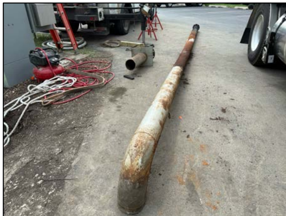
Photo showing old metal piping.
