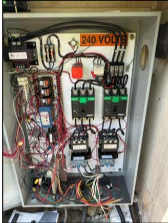
Photo showing old Waterford Panel.
