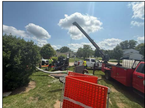
Bypass at Waterford Lift Station.
