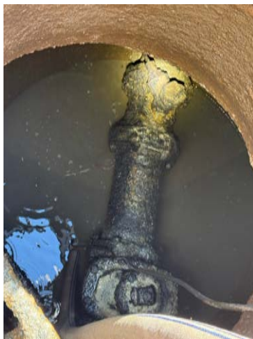
Faulty ARV on 8" forcemain associated with LS1.
