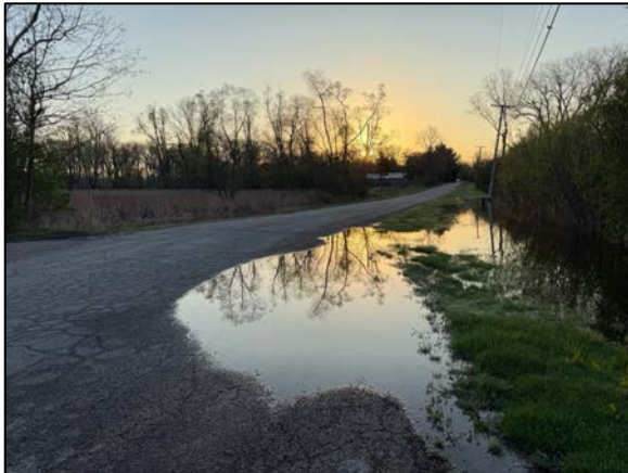
Local flooding on Timber Trail near plant.
