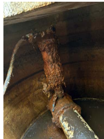
Faulty ARV on 8" forcemain associated with LS1.
