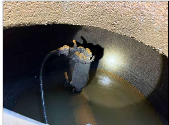
Faulty ARV on 8" forcemain associated with LS1.
