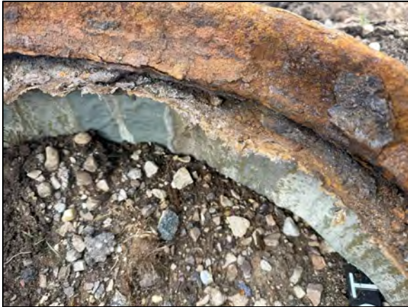
Photo of deteriorating manhole lips.
