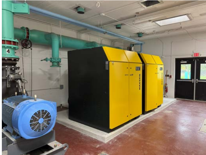
Two new Kaeser Blowers set on equipment pad.
