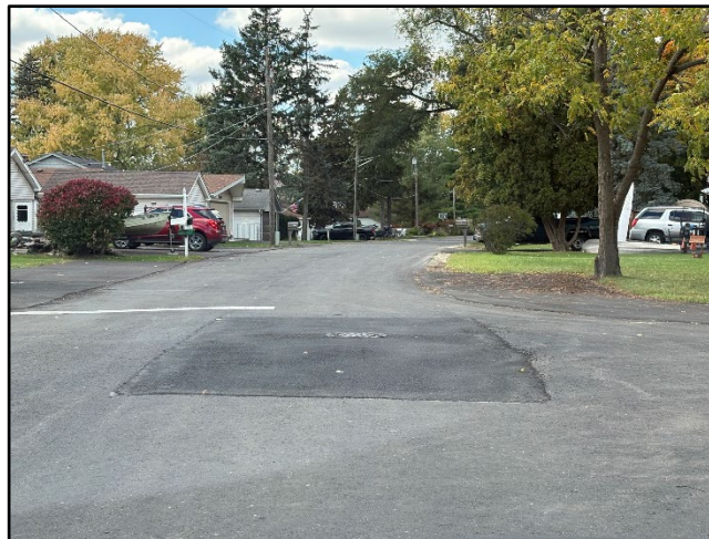
Patchwork around a manhole
