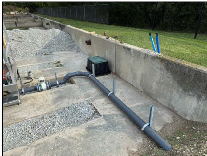
Septage Receiving Station piping and flowmeter location.
