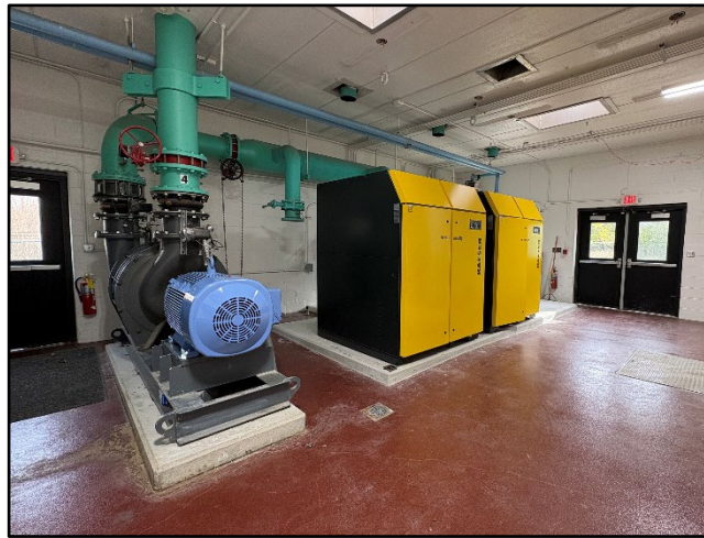
Two Kaeser Blowers placed on equipment pad
