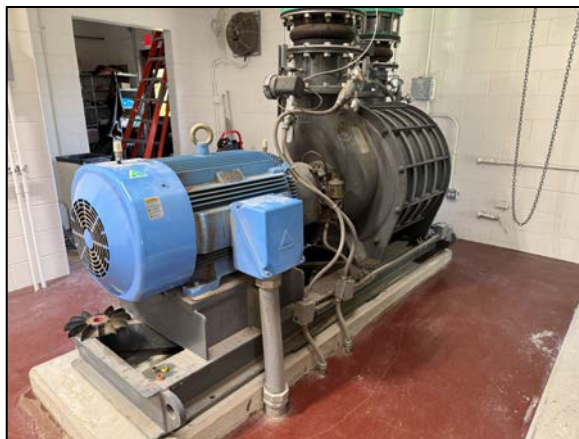
Photo of old motor. See fan on skid after melting.
