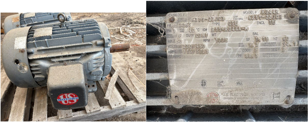
8. U.S. Motors Emerson Electrical Motors - Model #: R044A -Type: ID #: B11-R044A-M
