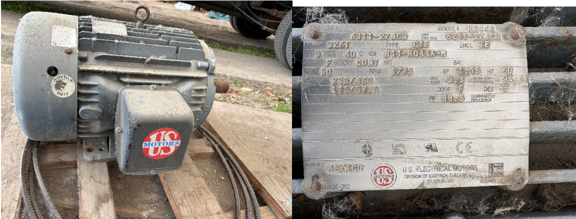
7. U.S. Motors Emerson Electrical Motors - Model #: R044A - Type: ID #: B11-R044A-M
