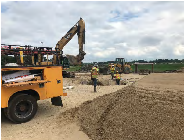
Service connections to the sanitary sewer mainline
