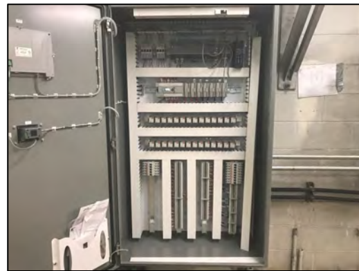
Interior of Dewatering SCADA Panel
