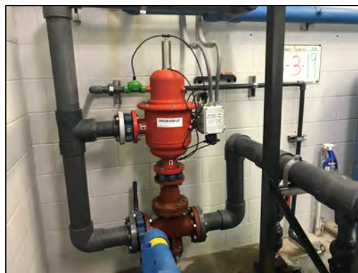
Strainer installed in NPW pump room.
