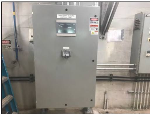
Dewatering Building SCADA panel.
